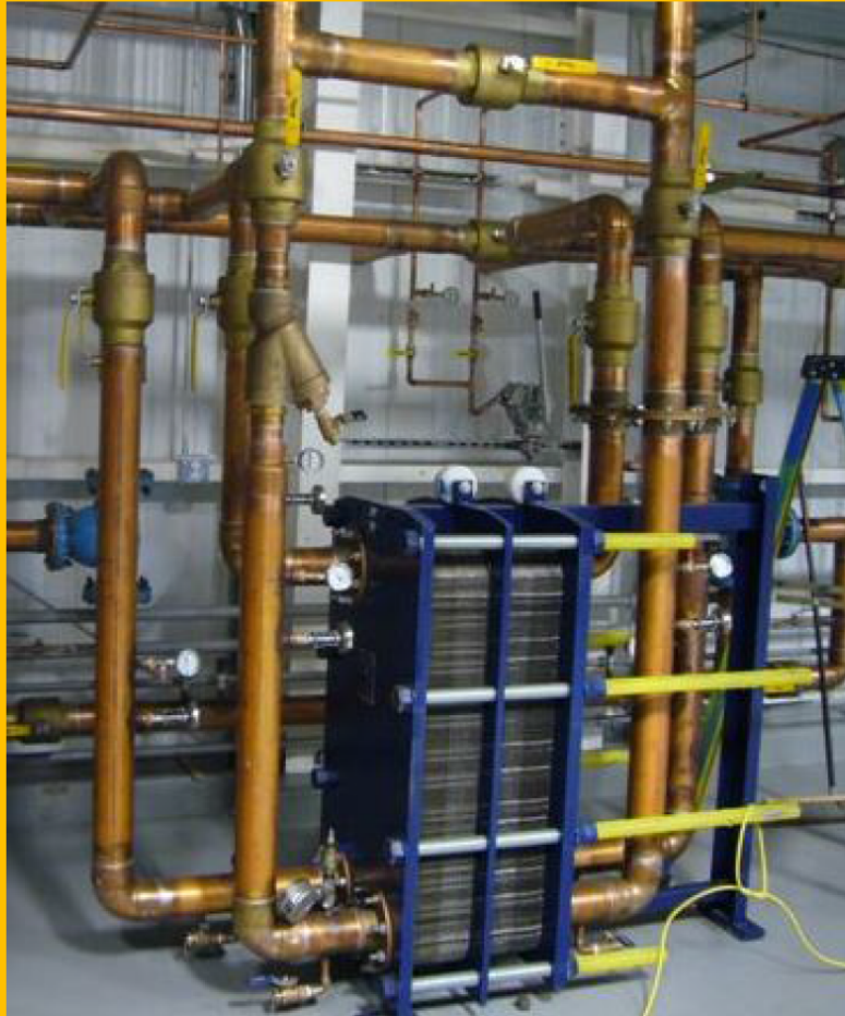
Plate & Frame Heat Exchanger
