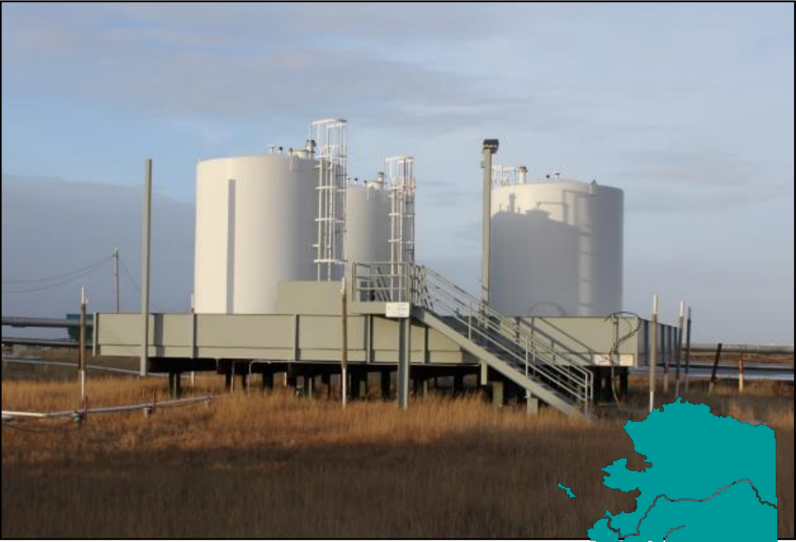
Kwigillingok Bulk Fuel Facility
